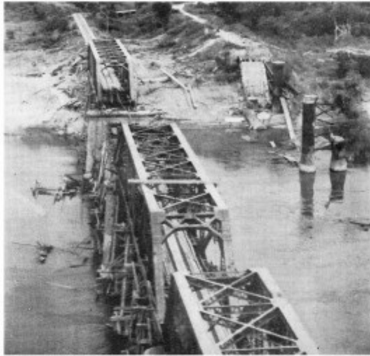
The Myitnge bridge after attack by RAF Thunderbolts. The bridge carried the main railway line from Mandalay to Rangoon
