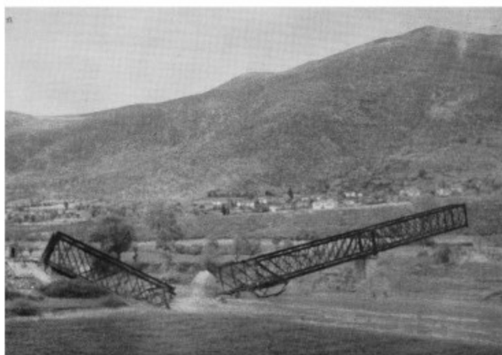
The Pinios railway bridge demolished by engineers of 19 NZ Army Troops Company
