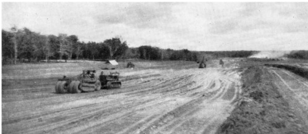
The bomber strip at Tebrau nearing completion by No. 1 Aerodrome Construction Squadron
