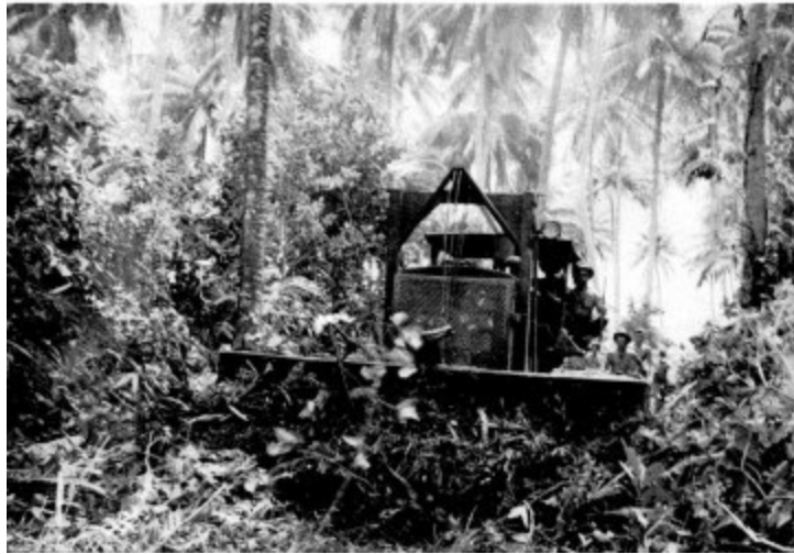
26 Field Company NZ Engineers forming a road though the jungle of Nissan Island
