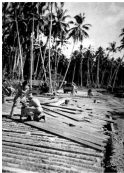
SOLID MAHOGANY PLANKS COVER A BRIDGE decked with coconut logs over Joroveto River, Vella Lavella. This was the work of 20 Field Company New Zealand Engineers.
